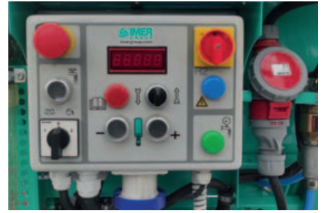
Display for diagnostic and operational indications
